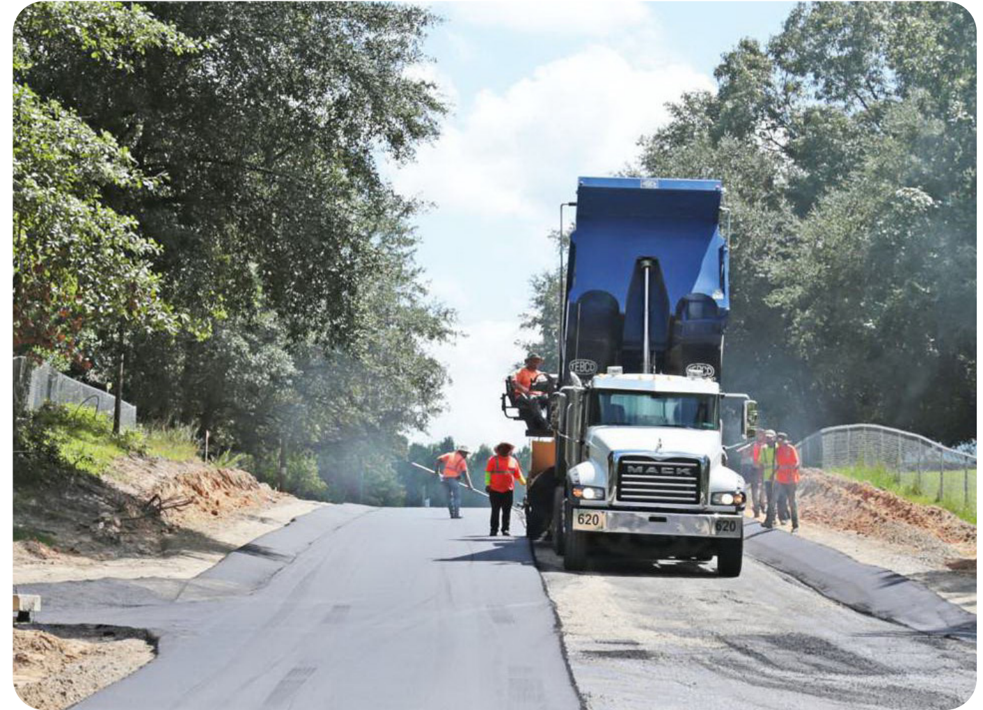
Photo: Road Paving on Peacock Dr. Funded by Sumter County Capital Projects Sales Tax
