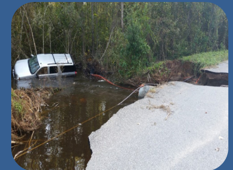
Photo: Flood Damaged Road in Sumter County
