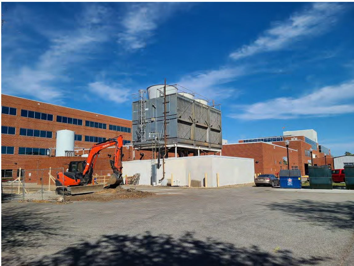
Above: View of the existing cooling towers in foreground with proposed new tower location in background
