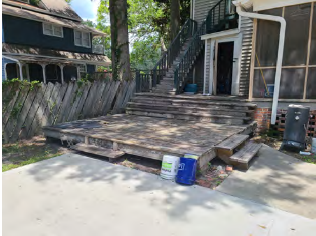
Existing deck to be removed and replaced
