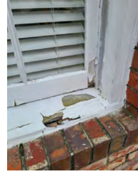
Example of damage to window sill on front façade.
