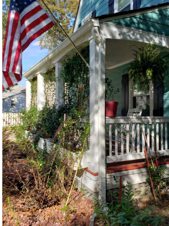
Front Porch Gutter (proposed for replacement)
