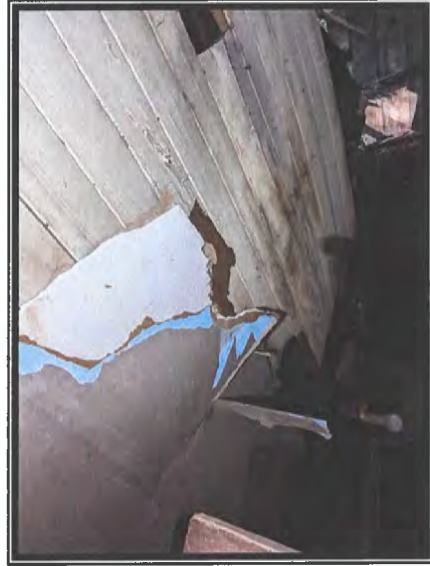
Photo #7 Asbestos Detected at 4% in Sheetrock System of Original House Footprint
