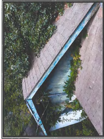
Photo #3 View Depicting Roof Area: Dark Gray Sealant at Chimney & Seams Contains Asbestos
