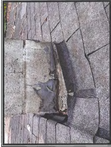
Photo #11 No Asbestos Detected in Chimney Flashing Sealant of the West Section
