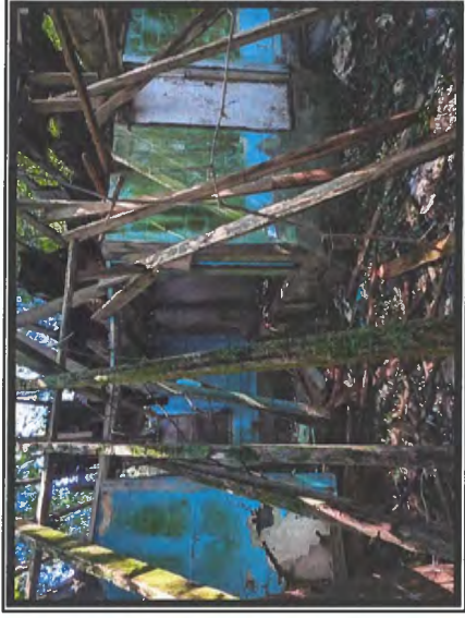
Photo #2 View Depicting the Collapsed Roof Structure
