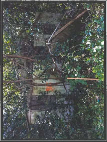
Photo #1 View from Franklin Ln. Depicting the Front of the CMU Block Structure
