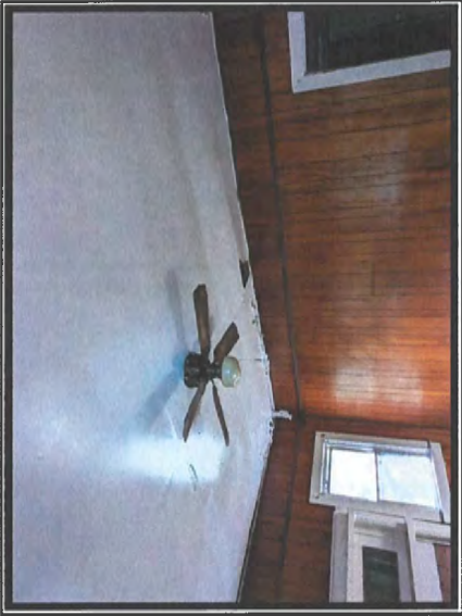
Photo #5 Asbestos Detected at 3% in Sheetrock Ceiling System, as Seen in Room 112A
