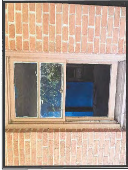
Photo #3 No Asbestos Detected in Glaze or Caulk Associated with Window Units
