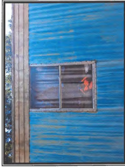
Photo #3 Asbestos Detected at 5% in Caulking Associated with Exterior Window Frames
