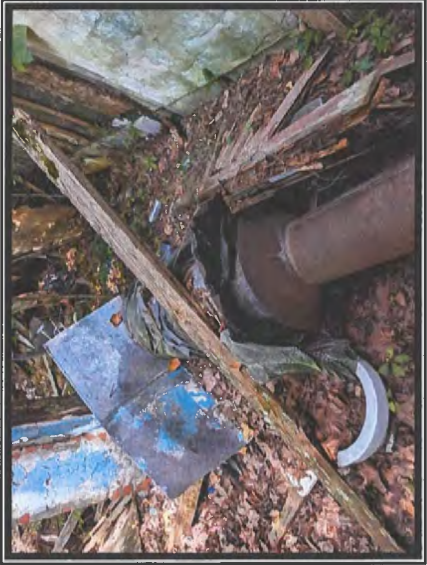
Photo #5 Asbestos-containing Roof Penetration Sealant Material in Debris of East Section
