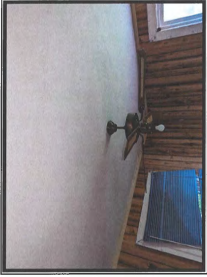
Photo #6 Asbestos-containing Sheetrock Ceiling in Room 112D
