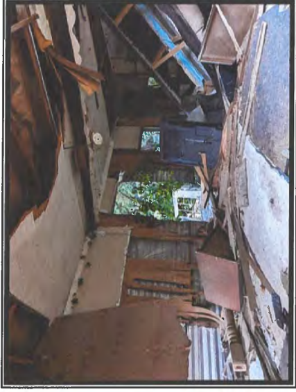
Photo #10 View Depicting Dilapidated State of the Mobile Home's Interior
