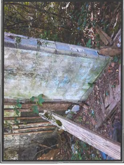
Photo #6 Remnant Areas of Asbestos-containing Wall Materials in East Section
