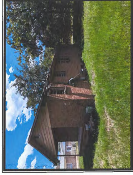
Photo #8 Southeast-facing View Depicting Damage to Roof Components
