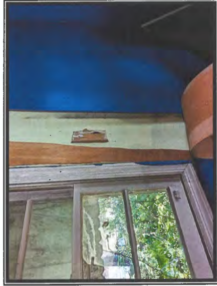
Photo #7 Asbestos-containing Sheetrock Wall behind Wall Paneling in Room 308A
