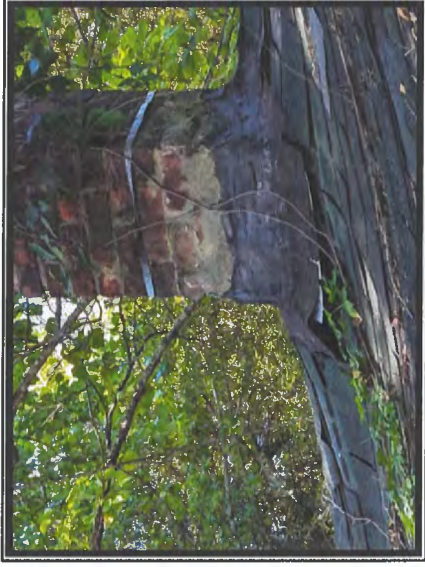
Photo #6 Chimney Flashing Sealant is Presumed to Contain Asbestos (PACM)
