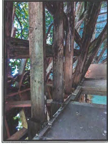
Photo #4 View Depicting Remnant Sheetrock Pieces on Wooden Ceiling Joists
