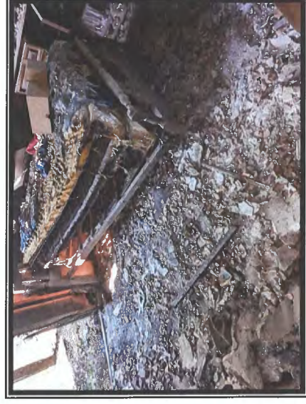
Photo #8 Asbestos-containing Ceiling Debris on Floor in Room 308F
