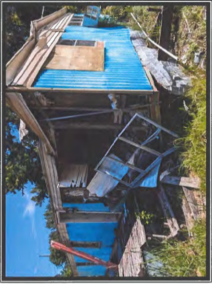
Photo #1 North-facing View Depicting the Damaged Condition of the Mobile Home
