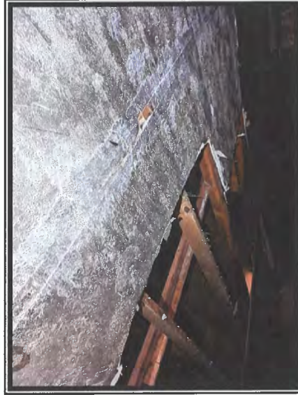
Photo #11 No Asbestos Detected in the Sheetrock Ceiling or Textured Material in the Addition Section
