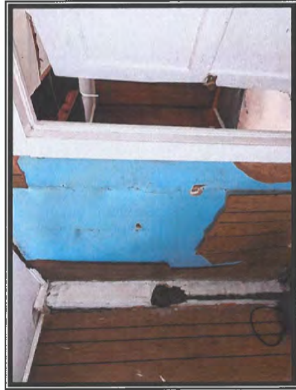
Photo #3 View Depicting Asbestos-containing Sheetrock Wall behind Wall Paneling
