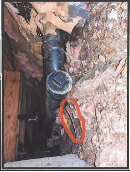
Photo #2 View Depicting Asbestos-containing Sheet Flooring Remnant on Ground in Crawl Space
