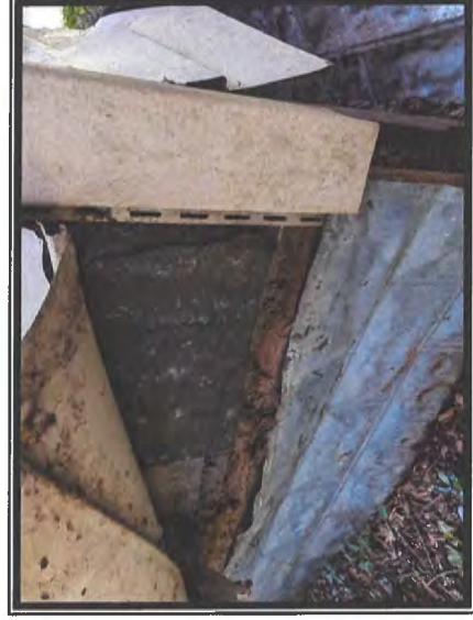
Photo #4 View Depicting Vinyl Wall Cladding over Sheathing Felt and Original Wood Panels
