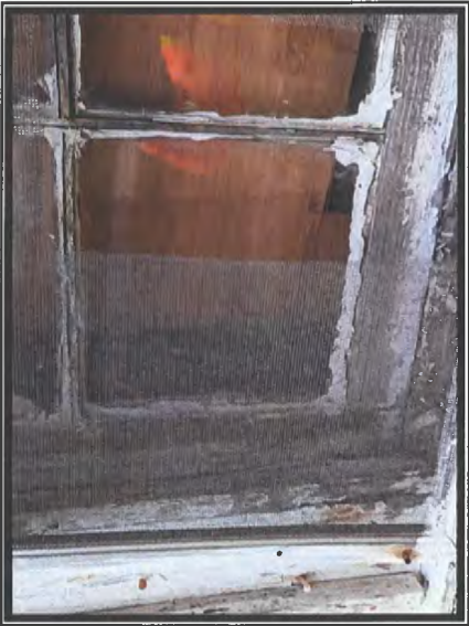
Photo #5 <1% Asbestos Detected in Window Glaze
