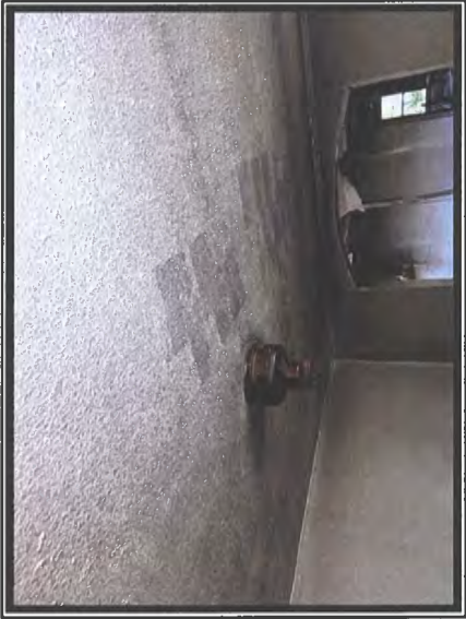
Photo #9 No Asbestos Detected in Spray-applied Ceiling Texture (Sheetrock is RACM)
