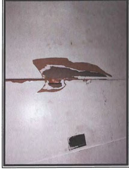
Photo #8 No Asbestos Detected in Gypsum Wallboard Panels
