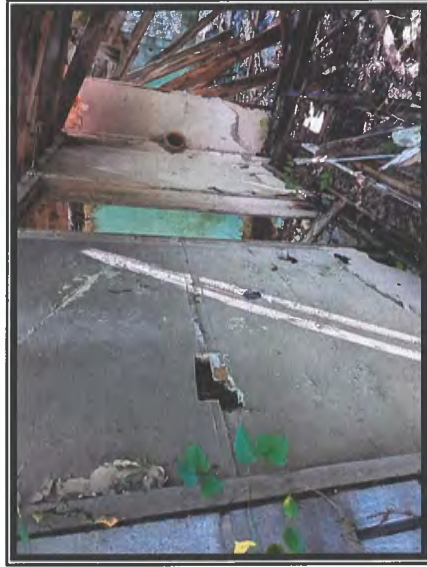
Photo #3 Remnant, Asbestos-containing Sheetrock Wall Section
