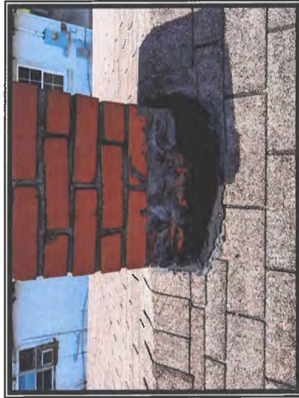
Photo #7 Asbestos Detected at 6% in Chimney Flashing Sealant
