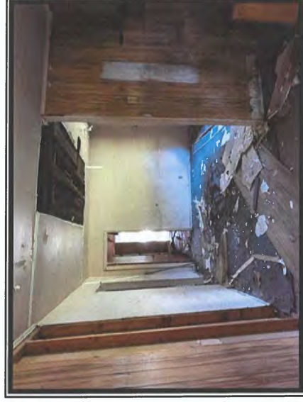
Photo #4 View Depicting Dilapidated Interior Conditions
