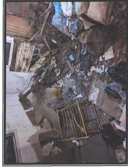
Photo #8 Asbestos-containing Sheetrock Wall & Ceiling Debris Scattered in Room 22B
