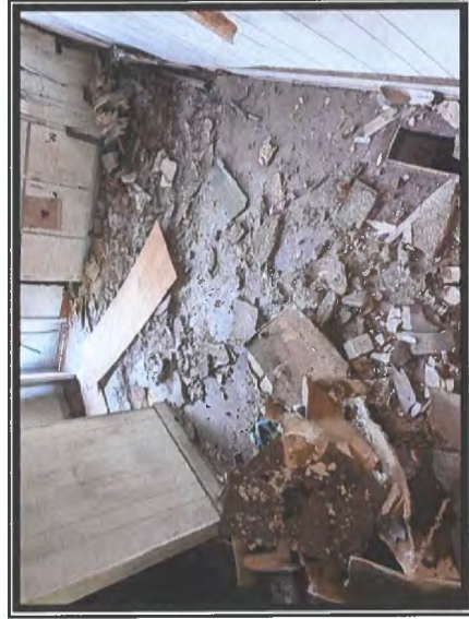
Photo #11 Asbestos-containing Sheetrock Ceiling Debris on Floor of Room 308E
