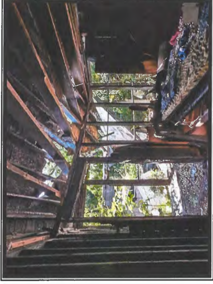
Photo #6 View Depicting Significant Fire Damage to Building Materials in Room 308F
