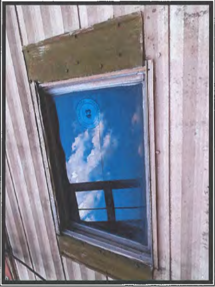
Photo #5 Asbestos Detected at 5% in Tan-colored Window Frame Sealant Material
