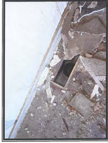
Photo #12 No Asbestos Detected in Duct Tape Associated with Vent and Crawl Space Ductwork
